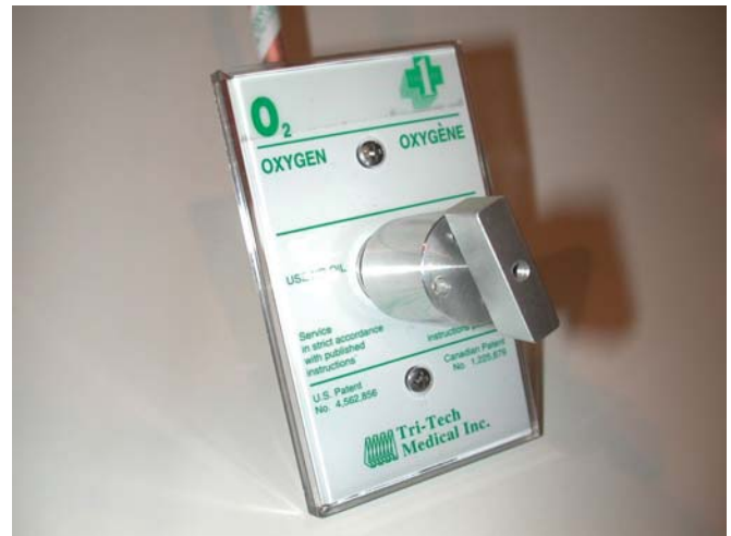
DISS Gas Outlet with DLO Locking Device Installed and Key Inserted for device removal
